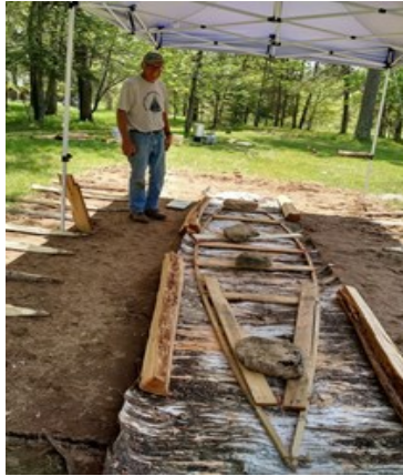
A construction frame is used to form the bark around. It will be removed later.
